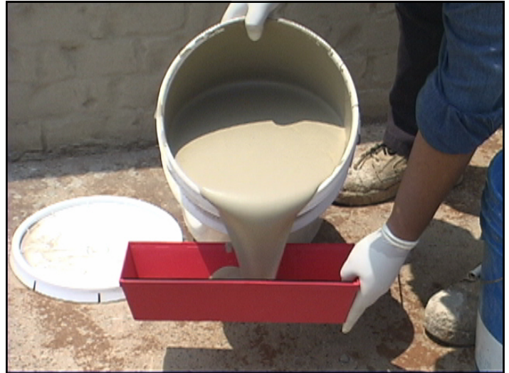
The finishing mix is poured into a mud pan where it will be quickly pulled onto the wall with a wallpaper brush.
